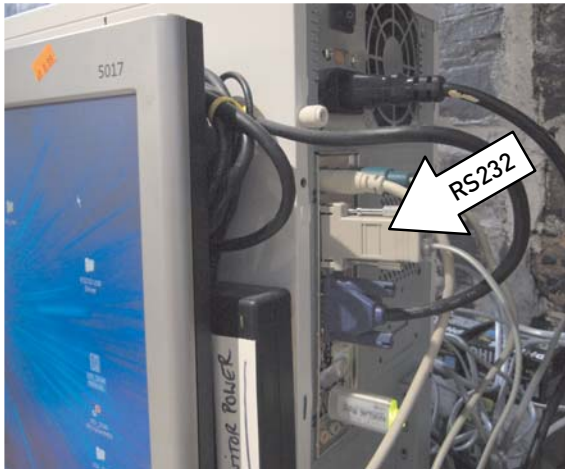
The RS232 connection for programming the LED sign is located directly above the blue monitor connection at the IDP's built-in PC.
